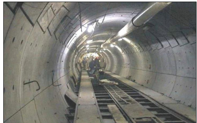
Fig. 2. Gallery of the HADES underground research facility (Mol, Belgium) lined with concrete wedge blocks.
