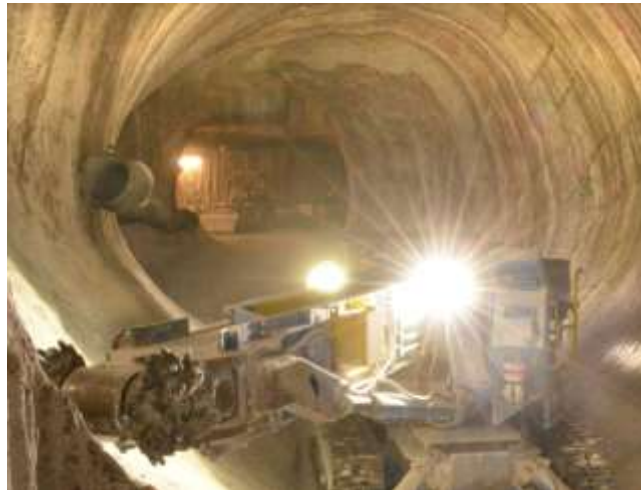
Fig. 4. Recutting of the rock salt profile at a site in the Asse II salt mine intended for barrier construction.
