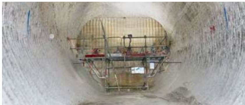
Fig. 12. Construction of a formwork wall shortly before completion for concreting an abutment.
