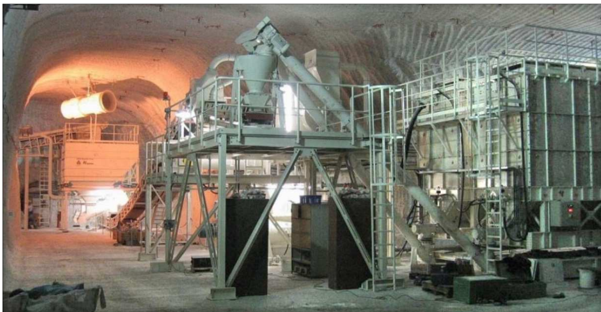
Fig. 7: Asse salt mine. Components of the pneumatic conveying system.
