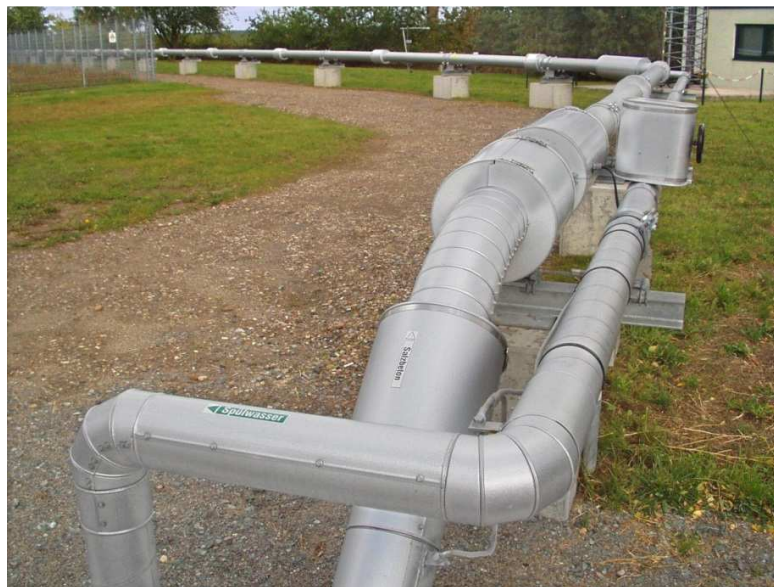
Fig. 3. Repository for radioactive waste Morsleben. Delivery and flushing water pipeline between the pumping station and the shaft. Both pipelines are insulated and equipped with a heating.
