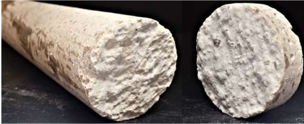
Figure 10 – Drill core from vertical drilling in the center of the structure - separation surfaces of the upper concreting joint.
