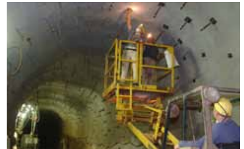
State of the art in constructing drift support systems in clay; the photo shows the roof bolt-shotcrete support system in the Konrad repository (Photo: BfS)
