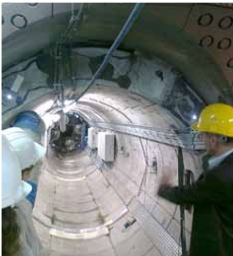
Connecting gallery of the HADES underground research laboratory (Belgium) (Source: ONDRAF/NIRAS).
