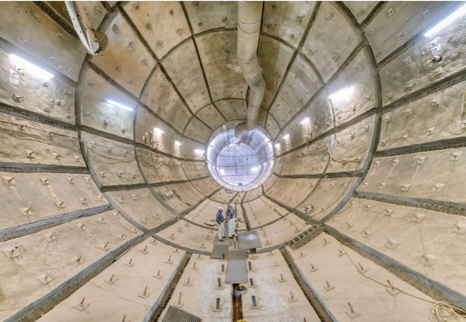
Konrad mine: Support in the area of the backfill processing plant on the 3 rd level
