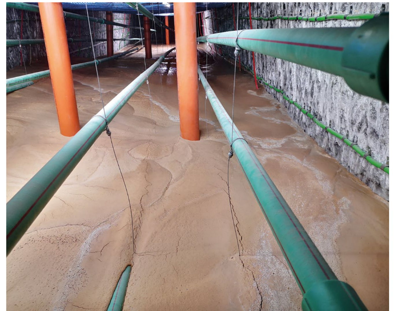
Concreting the lower half of a sealing structure in the Teutschenthal mine
