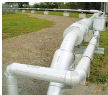
Injection and flushing water line of the stationary conveying plant Morsleben
