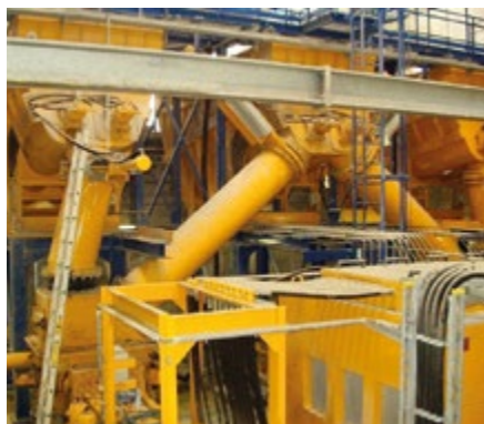
Storage tanks of the stationary conveying plant Morsleben with pipelines leading to the double piston pumps
