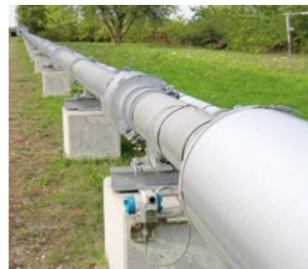
Injection and flushing water line of the stationary conveying plant Morsleben
