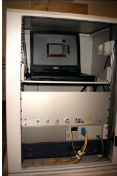
Fig. 3.76: Measurement rack with double FossFibreScan unit
