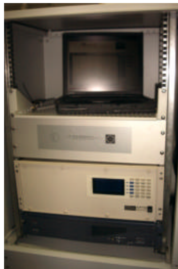
Fig. 3.77: Measurement rack with MOI interrogation system. MOI unit has been positioned after blind panel.
