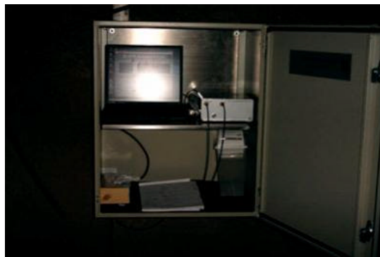
Fig. 3.56: Complete system installed in an industrial rack against the mine wall.
