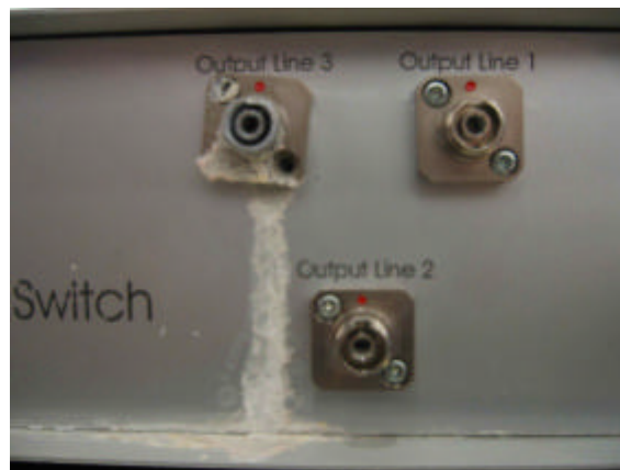
Fig. 3.32 Optical switch water intrusion
