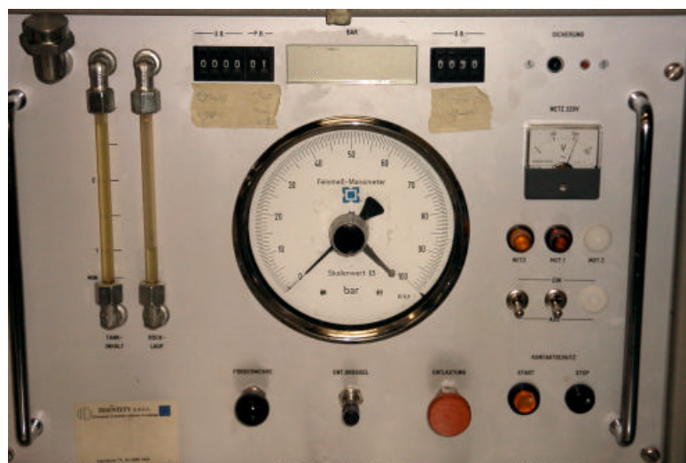
Fig. 1.36: Automatic pressure pump
