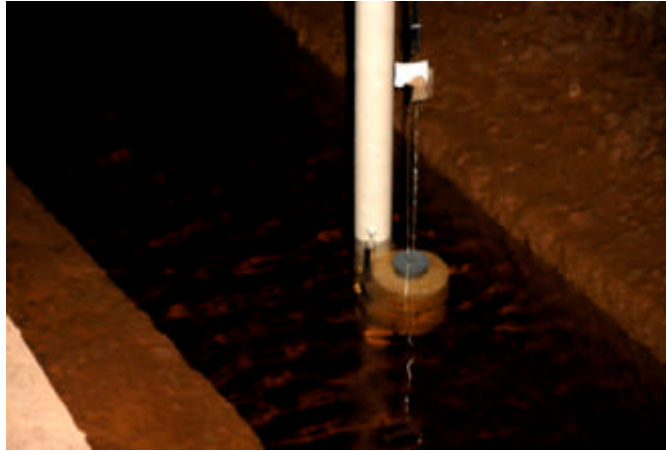
Fig. 3.54: Installed pH-head probe with filter to protect the reflectors against dirt in the drain water
