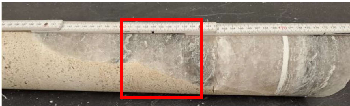
Figure 6 – Core sample of the contact area between concrete and formation obtained from borehole B20.
